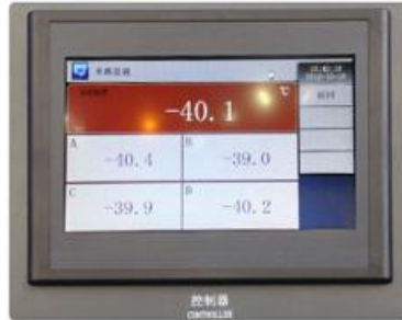
电池表面温度监控 Battery surface temperature monitoring
