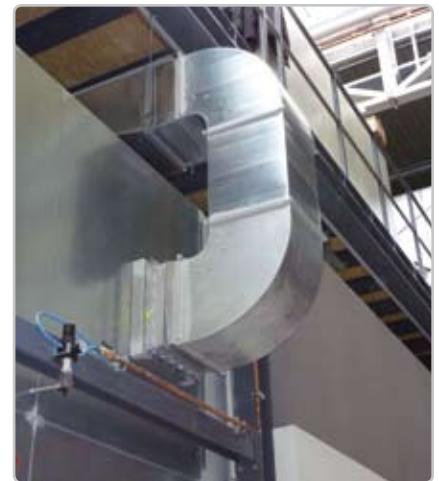
Direct connection to air conditioning system
